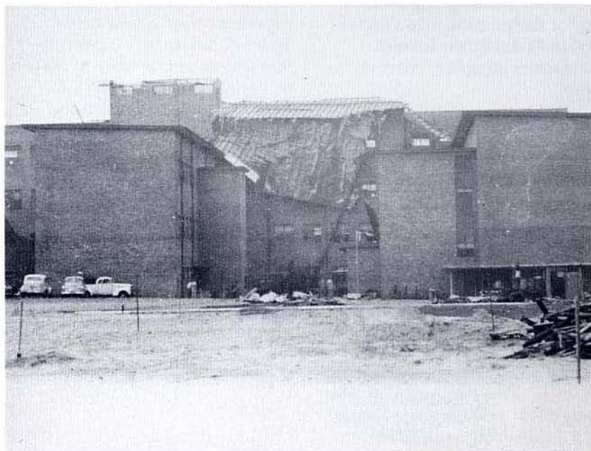
Storm damage to the roof of the Main Building, June 1956, an event frequently recalled by Kensington students of the day. (CN855)
