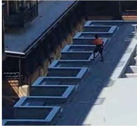
Lack of fall protection (i.e. harness) near roof edge
