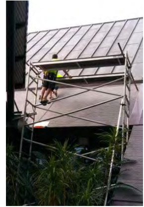
Scaffolding falls risk
