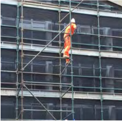
Scaffolding falls risk
