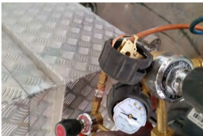
Damaged Oxy-Acetylene regulator in use on site
