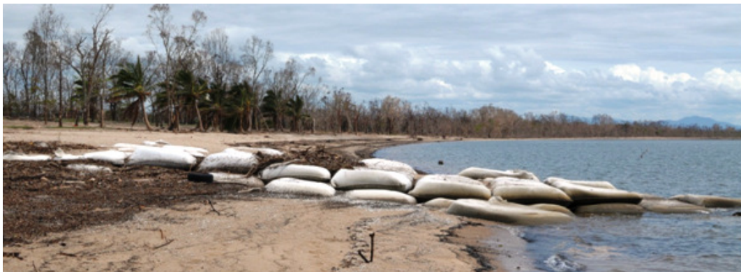
Figure 6: Cardwell Groyne (Qld) following TC Yasi
