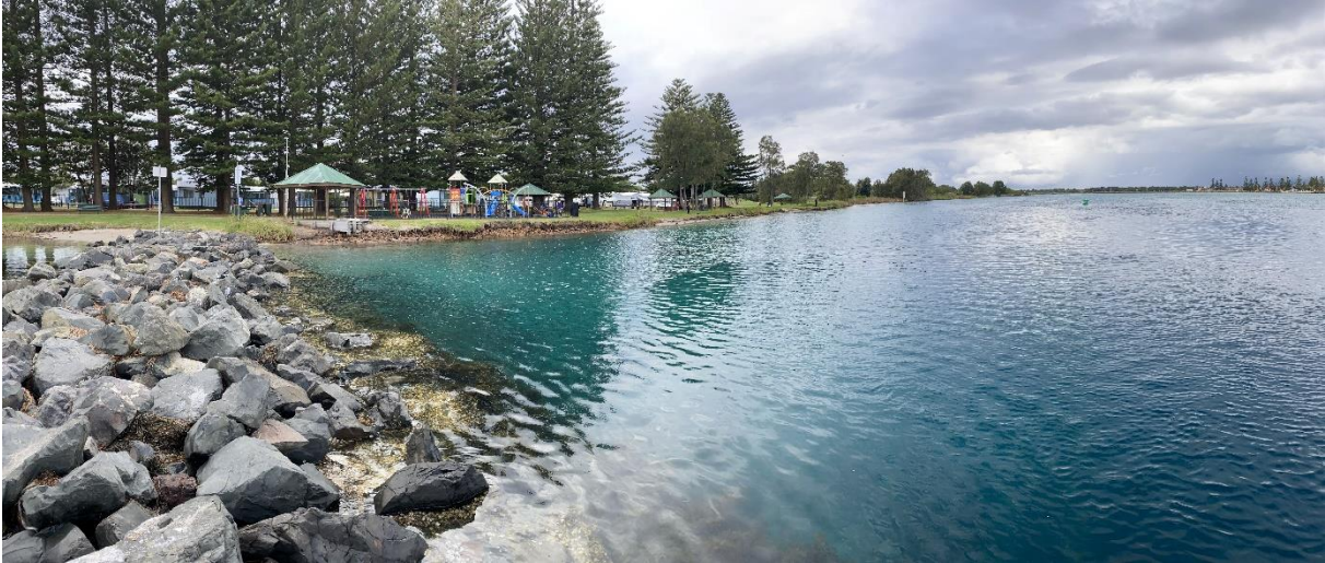
Figure 2.2 Erosion along the Windang foreshore as viewed from the end of the groyne
