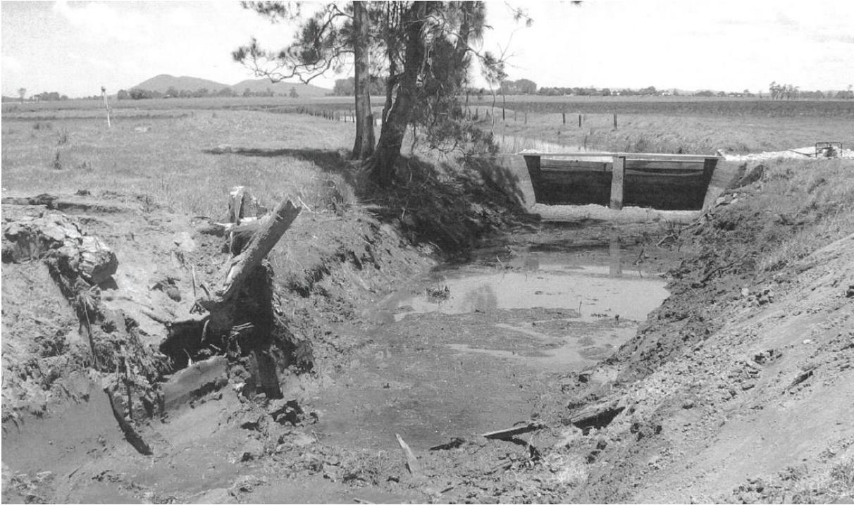
A.4: Drop boards on Kinchela No. 2 drain (Source: Ron Kemsely, Kempsey Shire Council)
