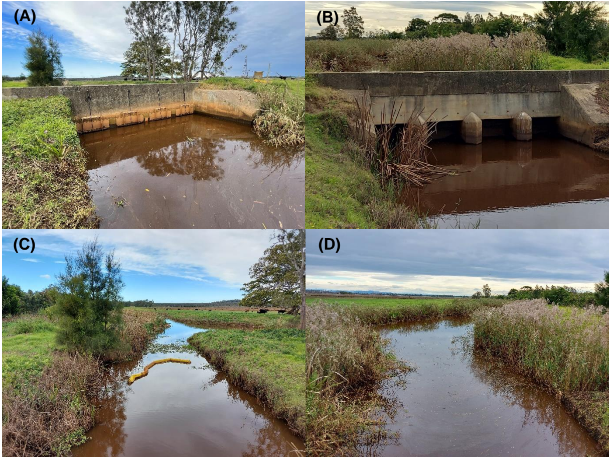
A.11: The Lock as inspected on 10 June 2021. Images are of The Lock from the downstream side (A) and upstream side (B) as well as on top of The Lock looking upstream (C) and looking downstream (D)
