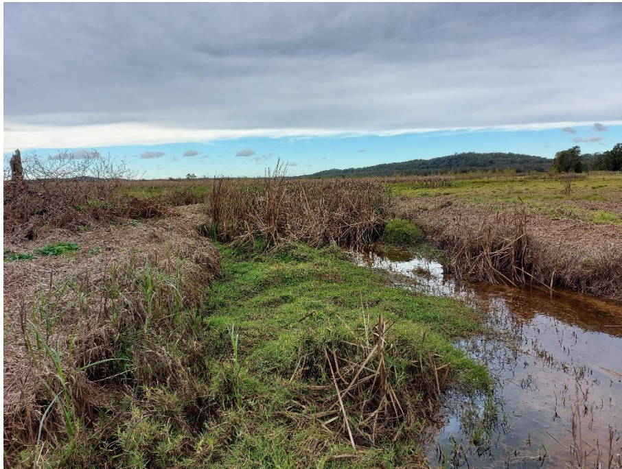
A.12: The remnants of North Drain weir as inspected on 10 June 2021
