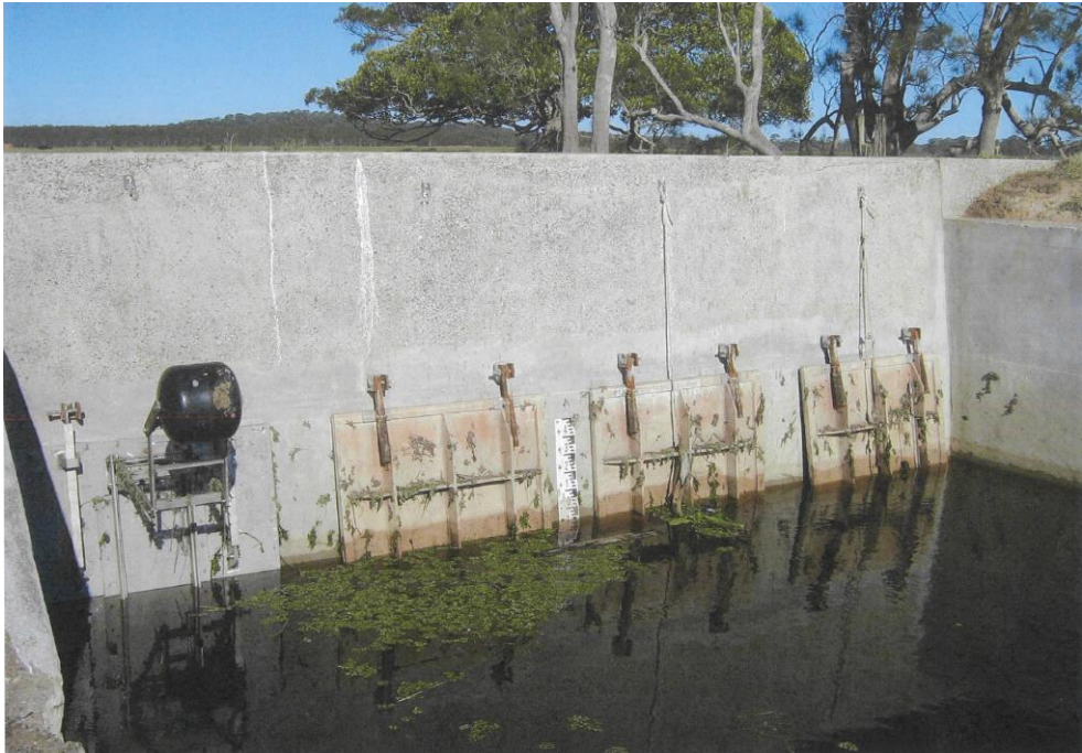
A.6: Buoyancy controlled auto-tide gate on The Lock (Source: Ron Kemsely, Kempsey Shire Council)
