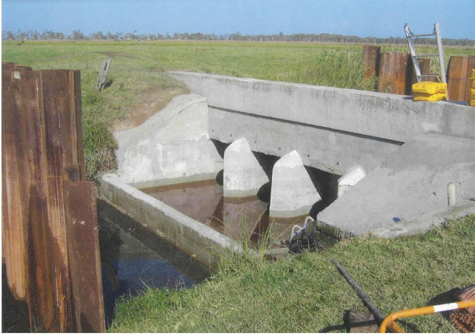
A.7: Wier constructed on the upstream side of The Lock (Source: Ron Kemsely, Kempsey Shire Council)
