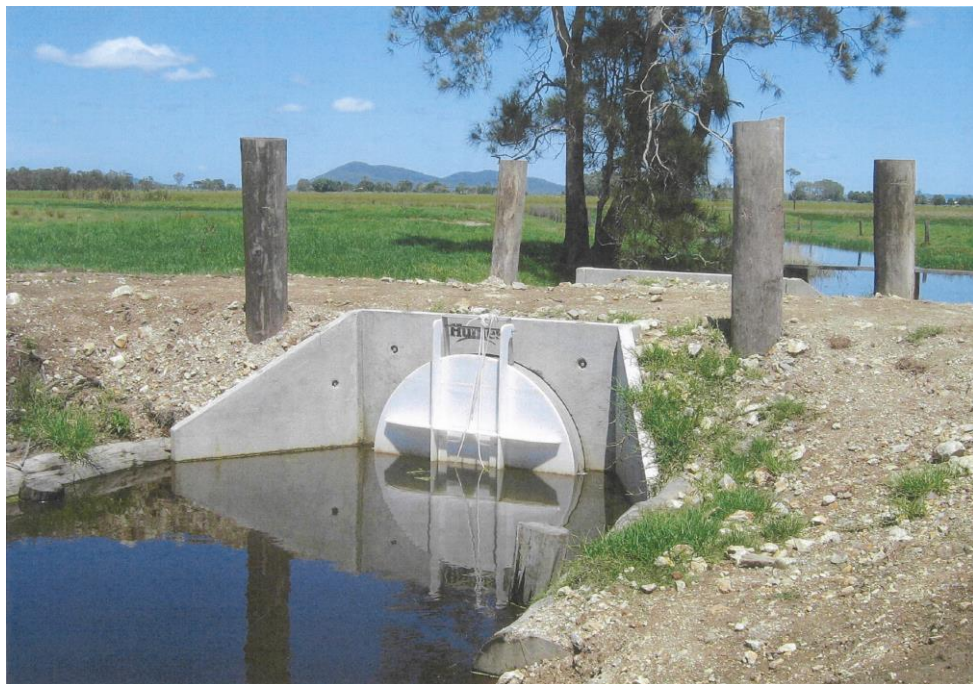
A.8: Floodgate on Kinchela No. 2 Drain (Source: Ron Kemsely, Kempsey Shire Council)
