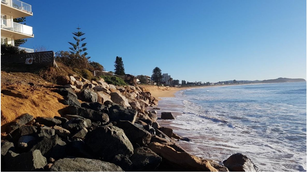
Figure 9: Erosion as seen from Wetherill Street looking north on 13 July 2018
