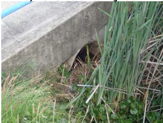
c) Blocked stormwater pit at southern end
