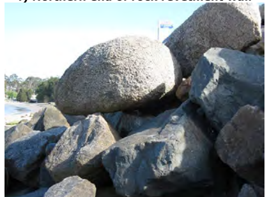
h) Example of precariously positioned rock
