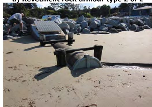
f) Stormwater outlet (blocked floodgate)
