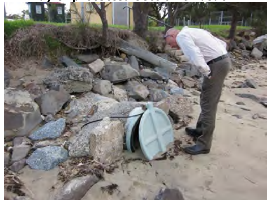
f) Stormwater outlet (blocked floodgate)
