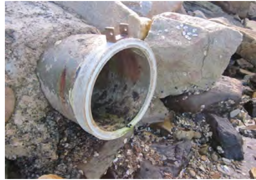
b) Stormwater outlet (missing floodgate)
