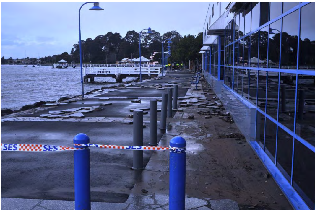
Figure 8-26: Inundation Damage to CBD Foreshore, 6 June 2012 (Mr Lindsay Usher)
