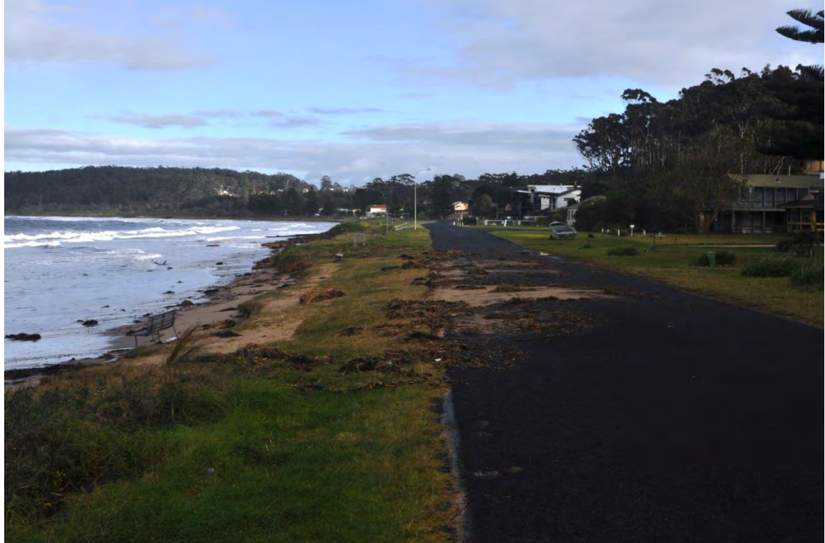
Figure 8-17: Overtopping of Bay Road, Long Beach, 6 June 2012 (Mr Lindsay Usher)
