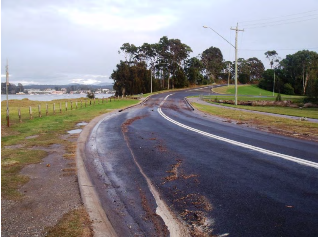
Figure 8-21: Overtopping of Myamba Parade at Surfside Beach (West), 6 June 2012 (Mr Dick Crompton)
