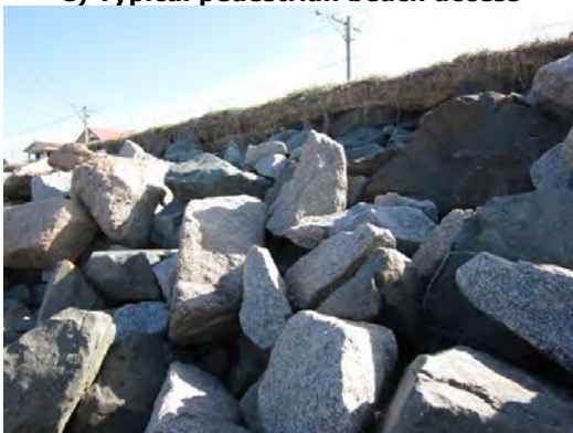
g) Some slumping of armour at the crest
