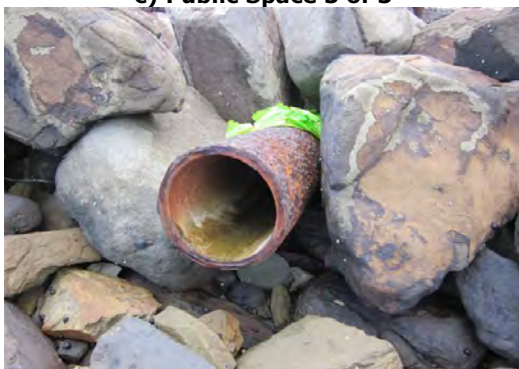
e) Typical local stormwater outlet
