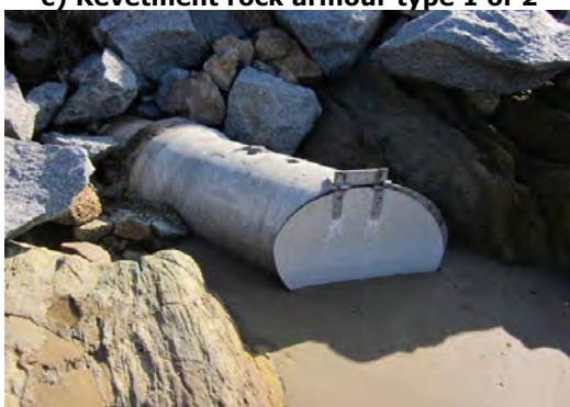
b) Stormwater outlet (blocked floodgate)
