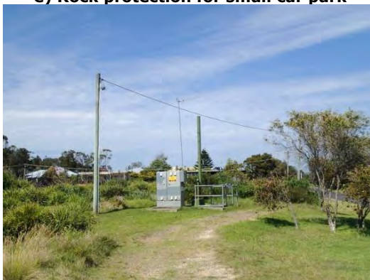
g) Sewage pumping station
