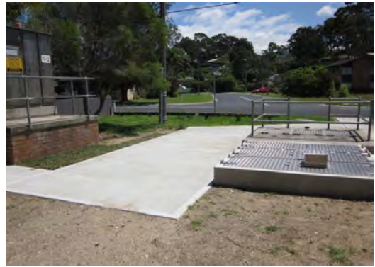
b) Sewage pumping station
