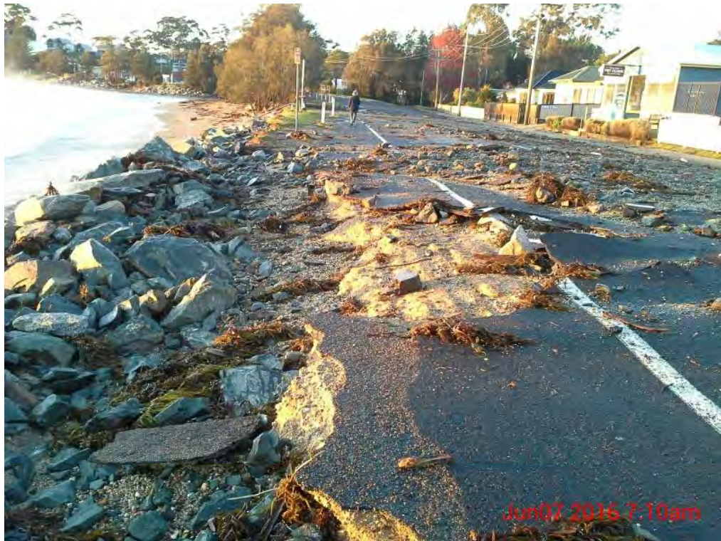
Figure 8-9: Post June 2016 Storm Damage to South of John Street (ESC, 2016)
