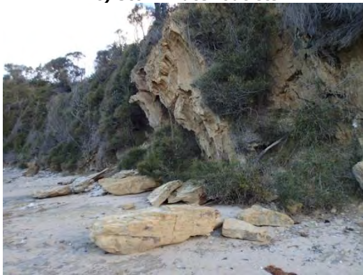
e) Backing rocky bluffs with rockfall
