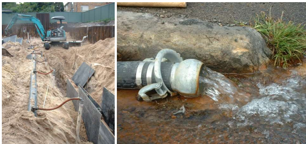
Figure 2.18: Groundwater dewatering in construction – Botany Sands aquifer. Source: Wendy Timms © Water Research Laboratory, UNSW.
