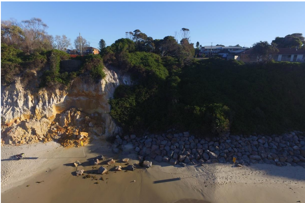
Figure 4-9: Photo of partial cliff collapse
