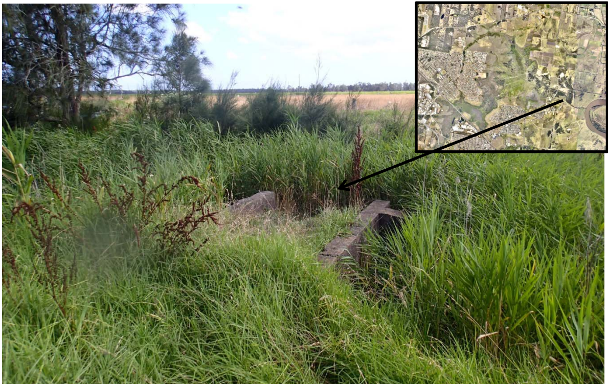
Figure 3.6: Collapsed culvert on side drainage channel, downstream of Woodberry Road
