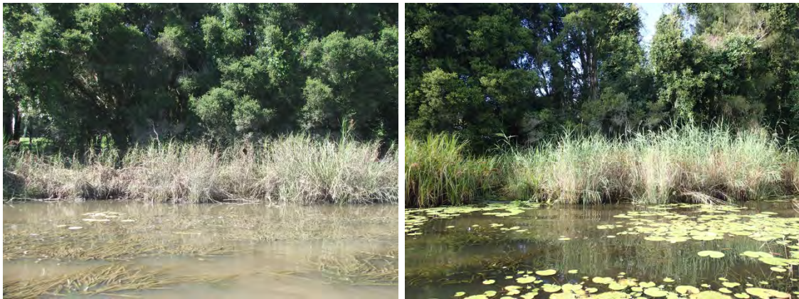
Figure 6-2: Riverbank Conditions Unchanged at L22B From 'Highly Resistant' in 2012 (Left) to 'Highly Resistant' in March 2015 (Right)
