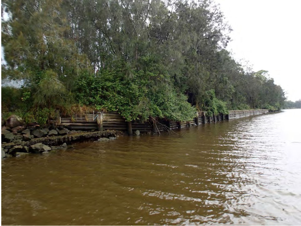
Figure 5-15: Armouring at Stretches L72 and L73 on the Lower Williams River (March 2015)
