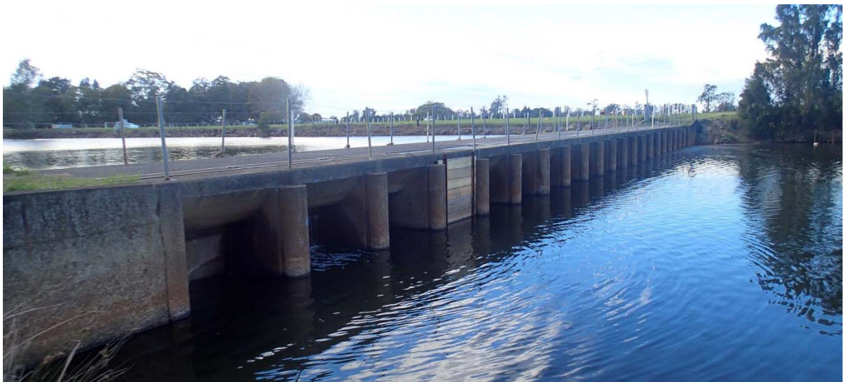
Figure 3.5: Clybucca Creek headworks (Menarcobrinni floodgates)
