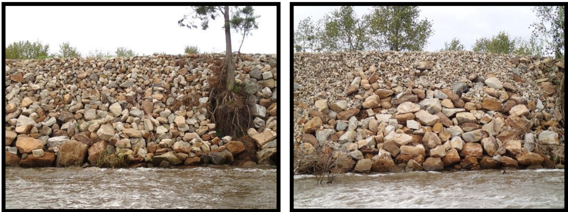
Figure 3-7: Armoring at Transects L63A and L63B
