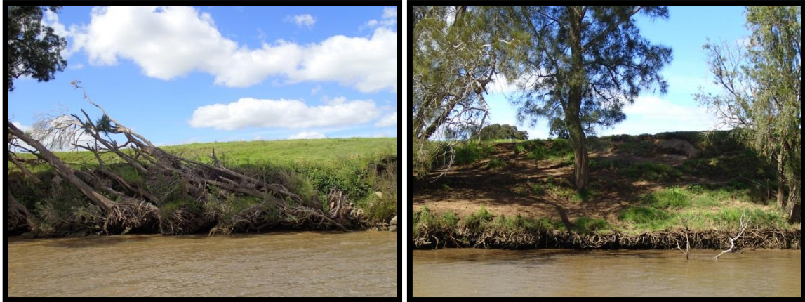
Figure 3-12: Significant Undercutting of Riverbanks with Stock Access Present at Stretches R54A and R63B
