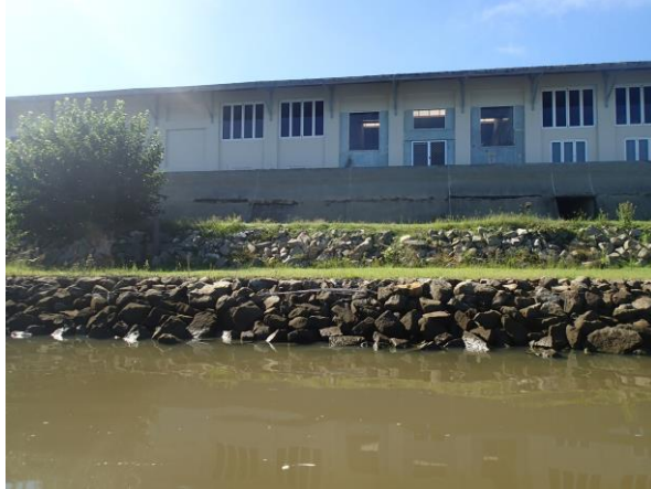
Figure A-3: Existing Rock Revetment Works and Concrete Seawall, Old Butter Factory (Ulmarra)
