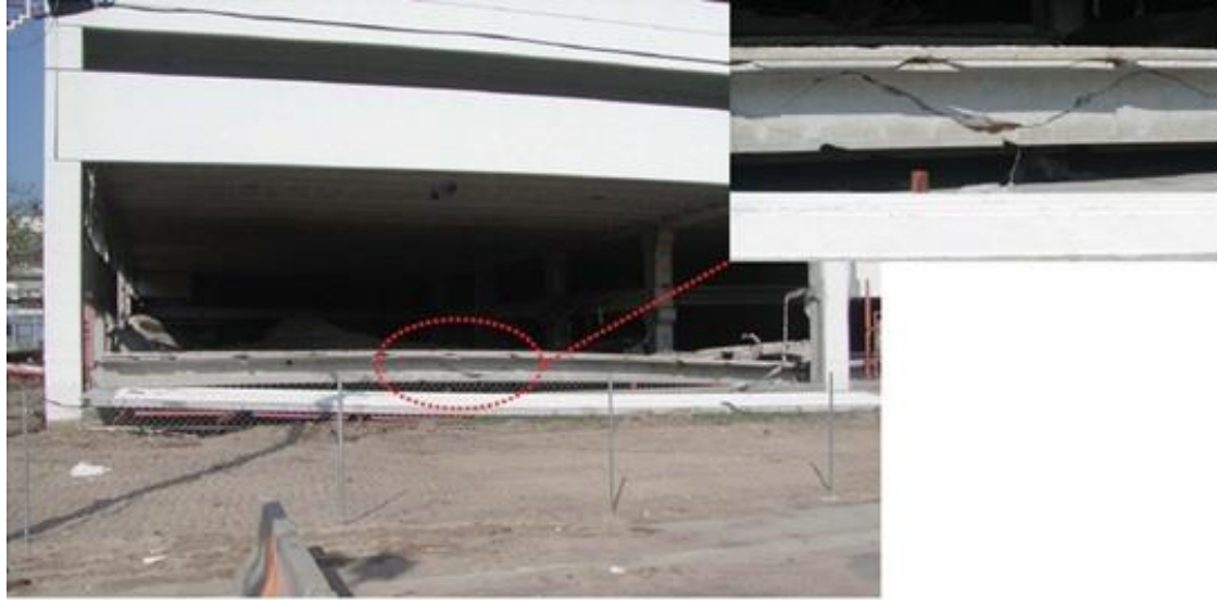
Figure 4-4: Structural damage due to uplift forces – Hurricane Katrina 2005 (Source: FEMA, 2012)
