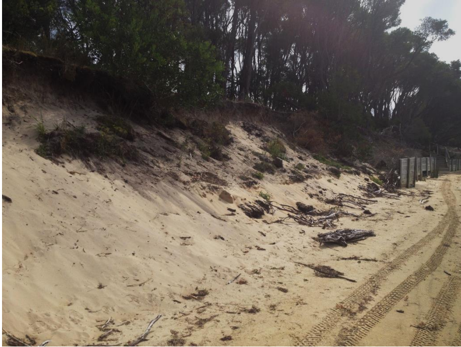
Figure 3.7: Eroded Foreshore at Western End of Seawall
