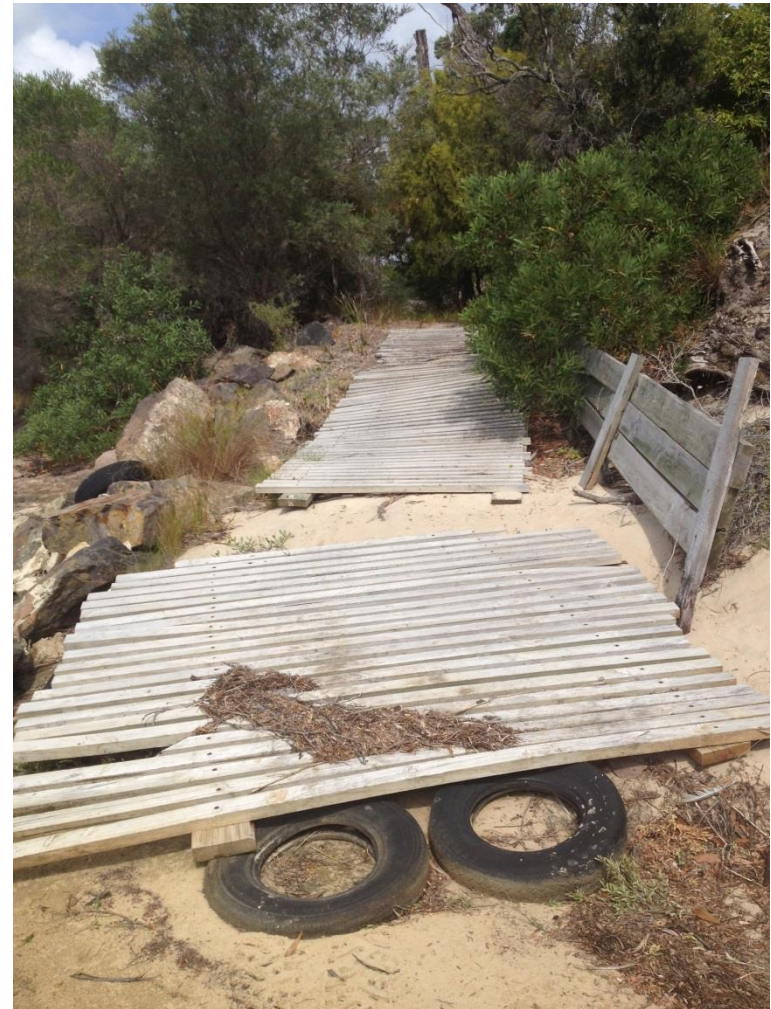
Figure 3.6: Damaged Timber Slatted Boat Ramp
