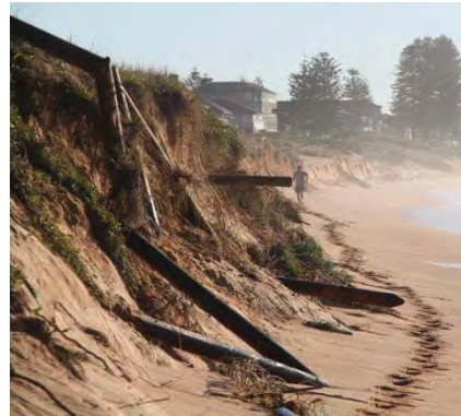
(b) Beach erosion at Narrabeen, 2011
