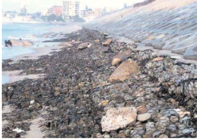
(a) Damaged gabions, Cronulla seawall, 1986
