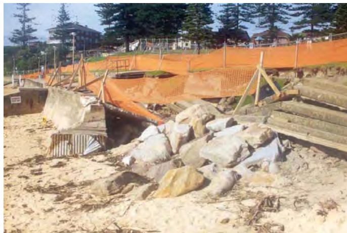
(b) Dee Why collapsed seawall, 1998
