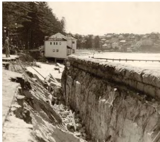
(c) North Steyne collapsed seawall, 1950
