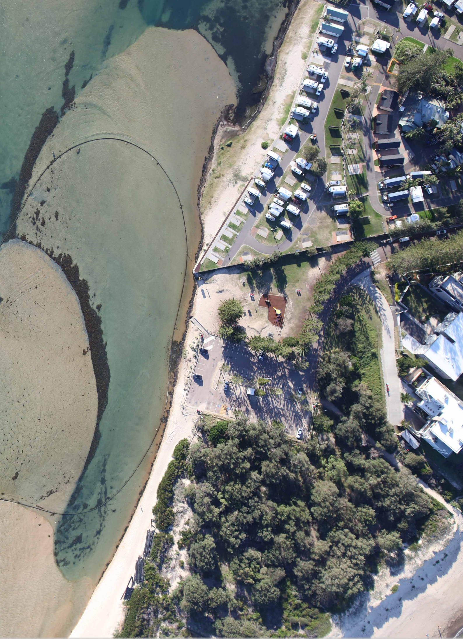
Drone view of dredging in the Lake Tuggerah estuary entrance channel, The Entrance, NSW; Photo: Chris Drummond, WRL, UNSW
