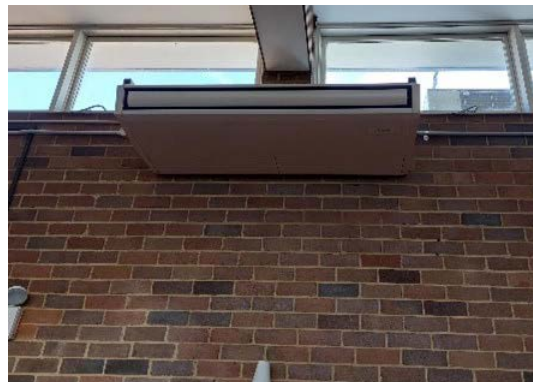
Figure 10. Position of the split units (interior and exterior).
