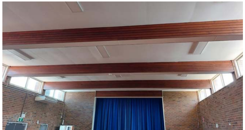
Figure 8. View of the ceiling with plasterboard panels in the main hall of the community centre. The windows on the perimeter are single-glazed without shading devices.
