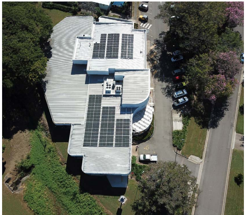
Figure 4. Installed solar panels on the Aitkenvale Library.
