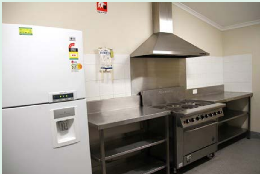
Fig. A5. Kitchen - appliances and hood.
