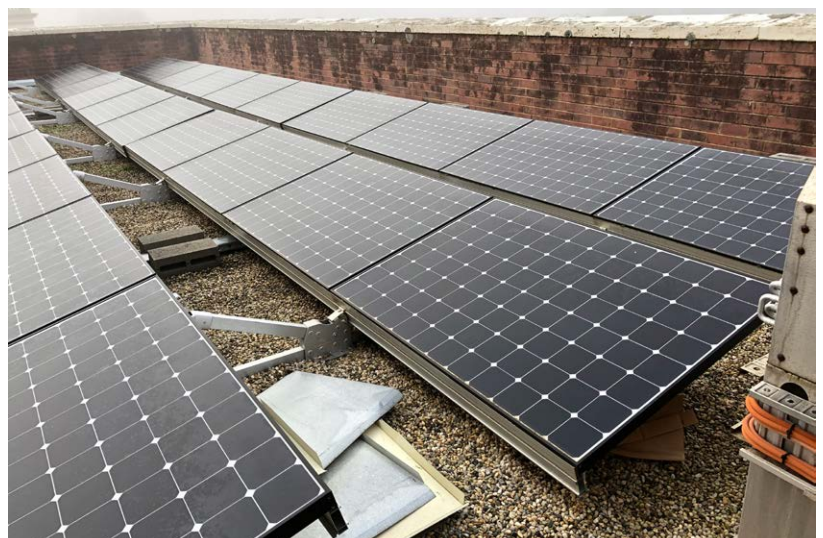
Figure 4. Installed solar photovoltaic panels.
