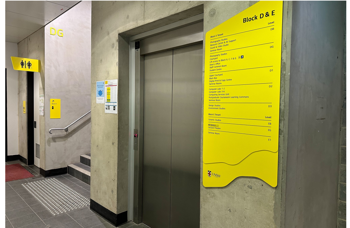
Elevator – Block D, Ground Floor
